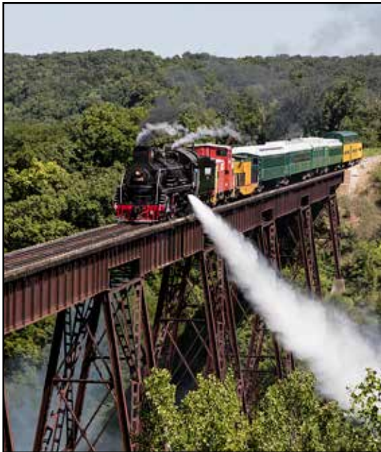
A Boone & Scenic Valley Railroad steam train crosses the Bass Point Creek Bridge.
